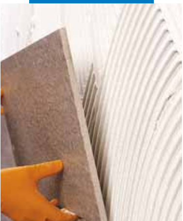
Laying large-sized, double-fired tiles on wall starting at the top and working downwards
